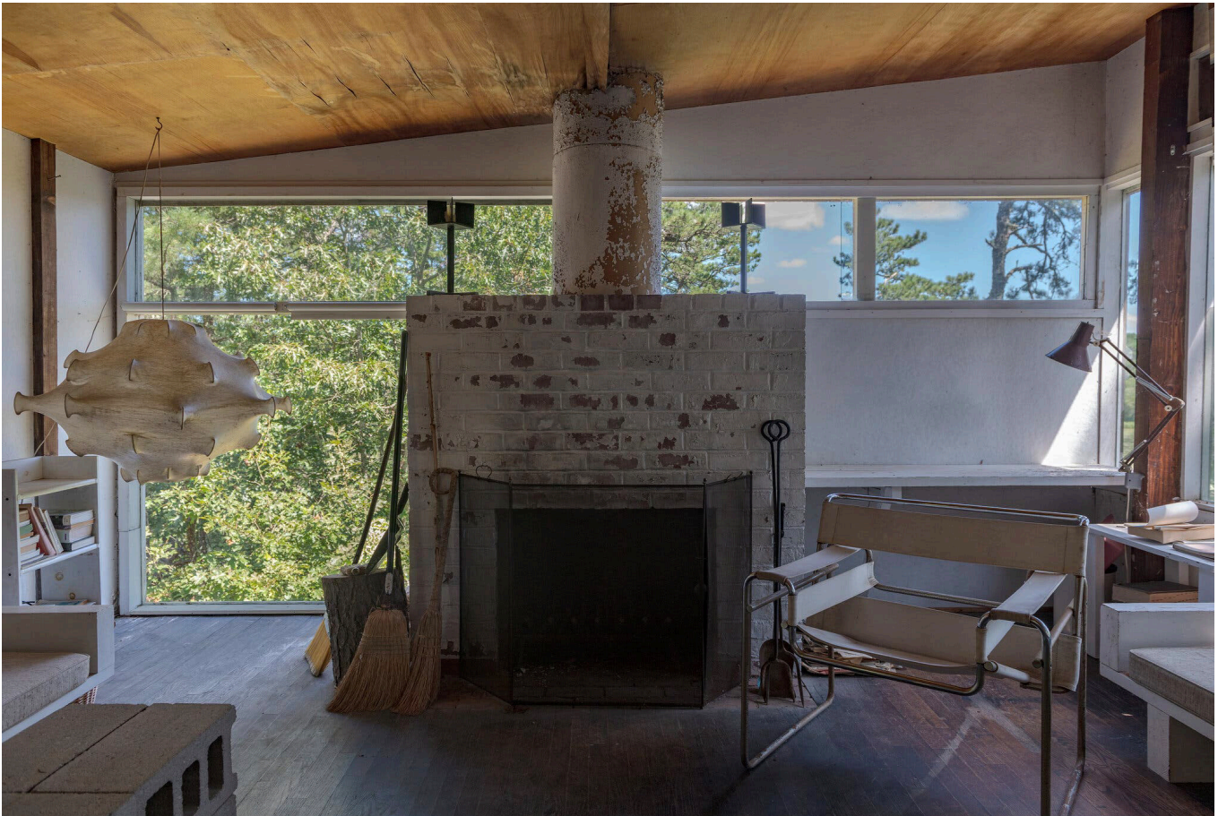
A leak in the roof has caused some damage to the birch plywood ceiling in the living room. The vintage lamp was designed by the brothers Achille and Pier Giacomo Castiglioni. Steven Smith for The New York Times
